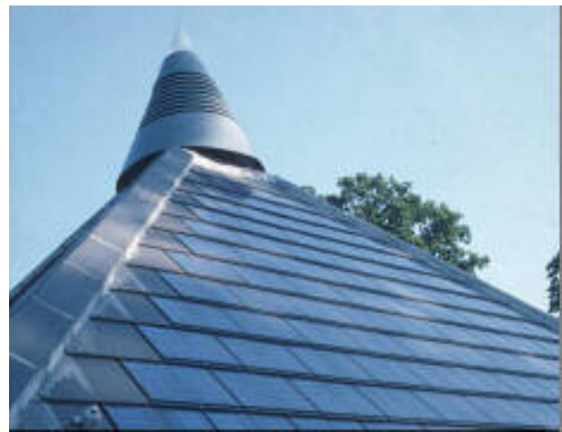
Figure 3. David Wilson Millennium Eco-House Showing PV Panels as Roof Tiles
