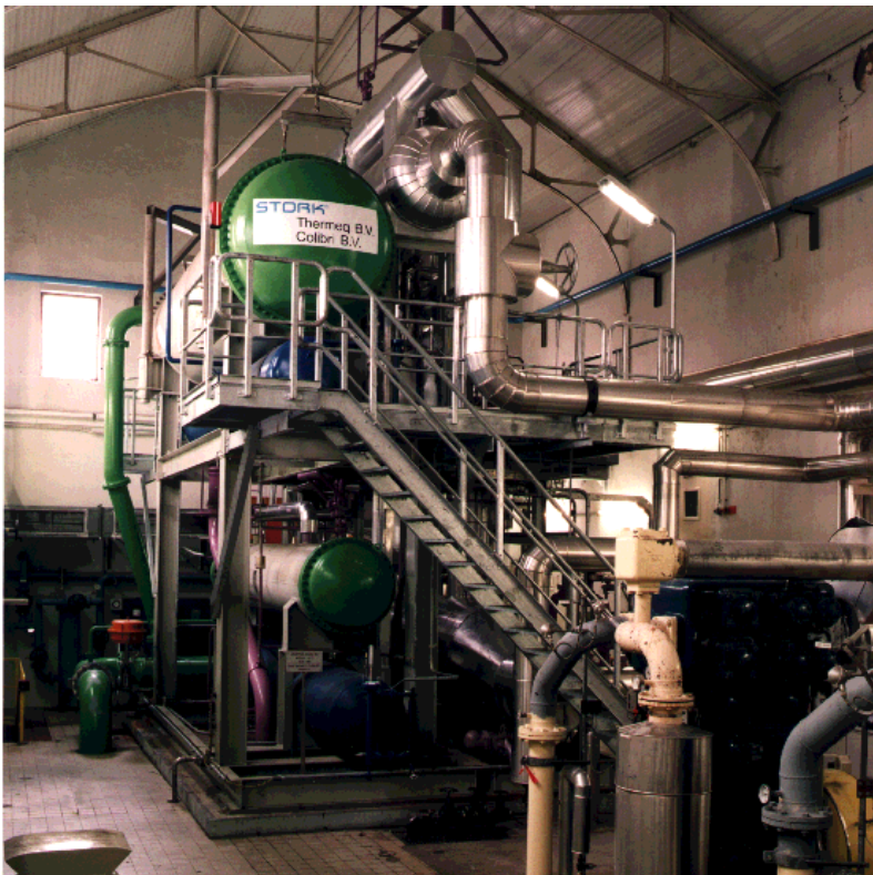
Figure 3 The ARP installed in a margarine factory in Rotterdam (Netherlands)
